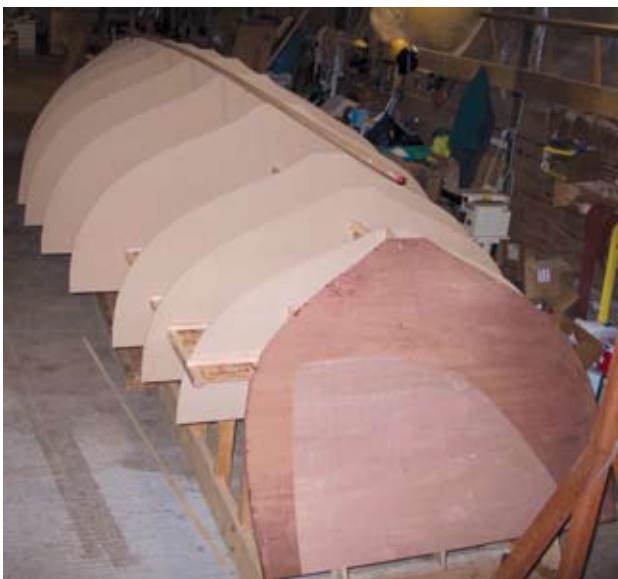
With the transom, laminated from 2 layers of 1/2" (12mm) marine ply, in place, we begin work to fit the inner keel or hog.
